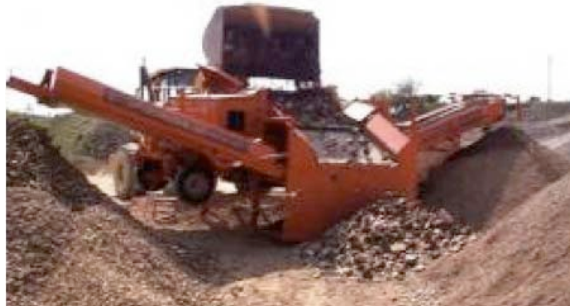
A primary screening feedstock for the removal of soil fraction and possible contaminants – plastics, paper, non-recyclables – before crushing.
